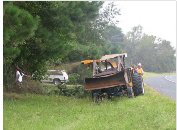
Figure 50. Photo. Removing brush as part of clear zone maintenance. Source: Texas DOT.
