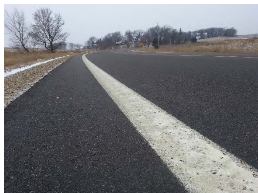
Figure 7. Photo. Delineation with enhanced (6-inch) edge lines.
