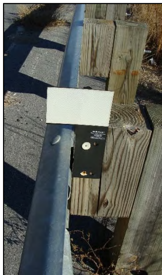
Figure 55. Photo. Delineators held in place with post bolts and installed on post.
