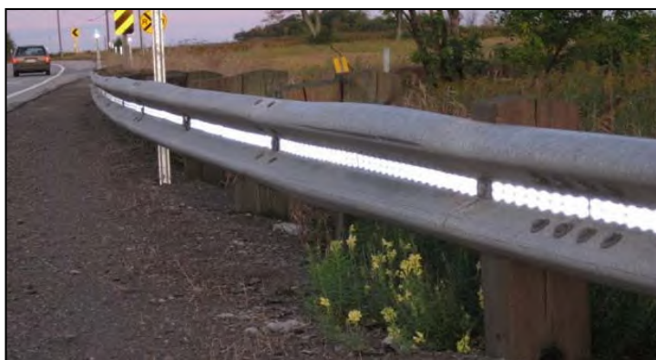
Figure 54. Photo. Retroreflective panels in the web of a W-beam. Source: Michigan DOT.
